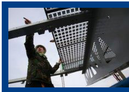
Soitec adds one of its new sun-tracking concentrated solar photovoltaic panels to the East Campus Utility Plant at UCSD. Engineer Luc Mader directs a crane operator. — Sean M. Haffey
